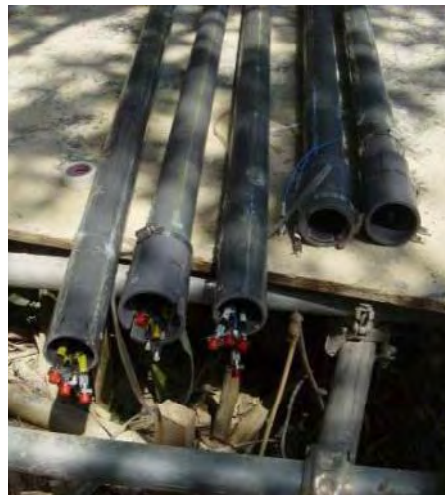
Slope Monitoring using Optic Fiber
